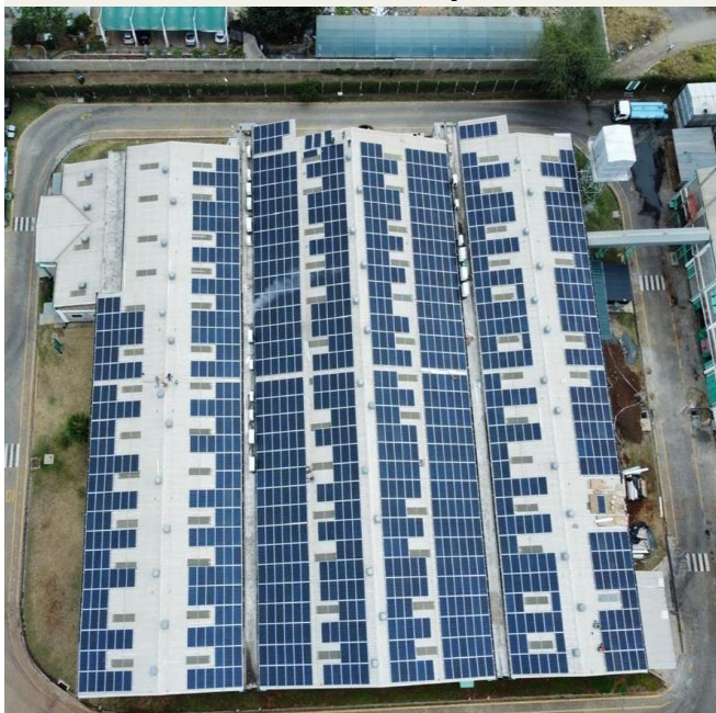
500 kWc roof mounted Nairobi, Kenya
